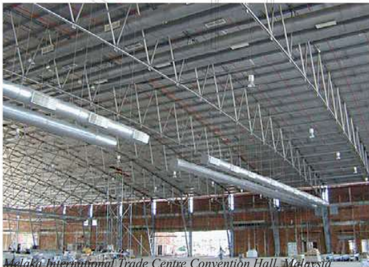
Melaka International Trade Centre Convention Hall, Malaysia 93.5m span stressed arch frame
