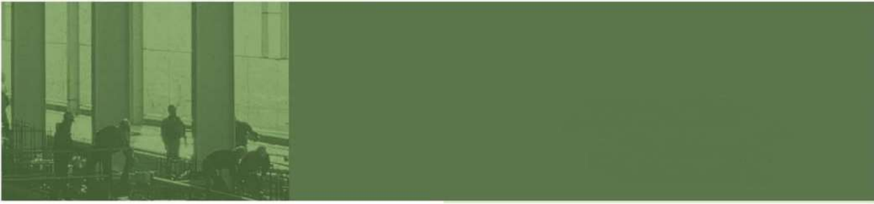
East Coast Economic Region, Kuala Terangganu Drawbridge- Heavy lifting of 2 nos skybridges
